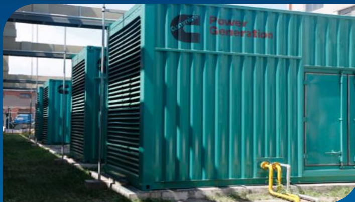
Outdoor cabin generator
