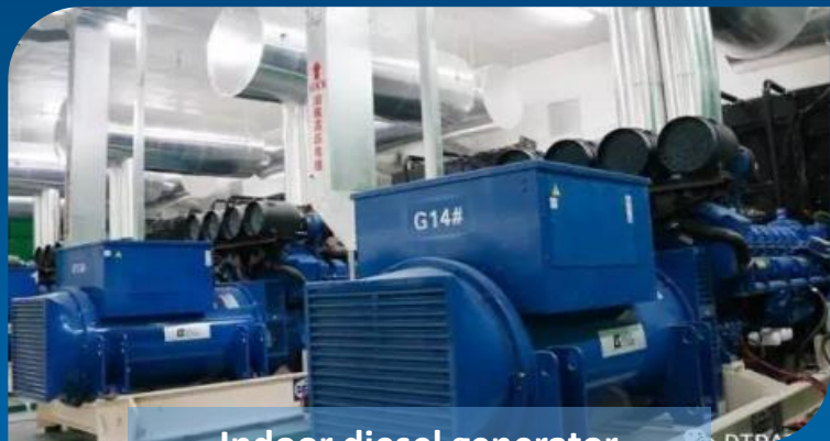
Indoor diesel generator
