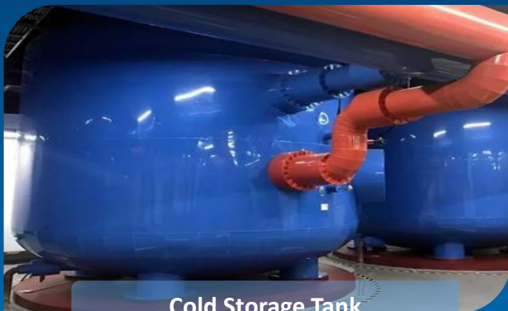
Cold Storage Tank
